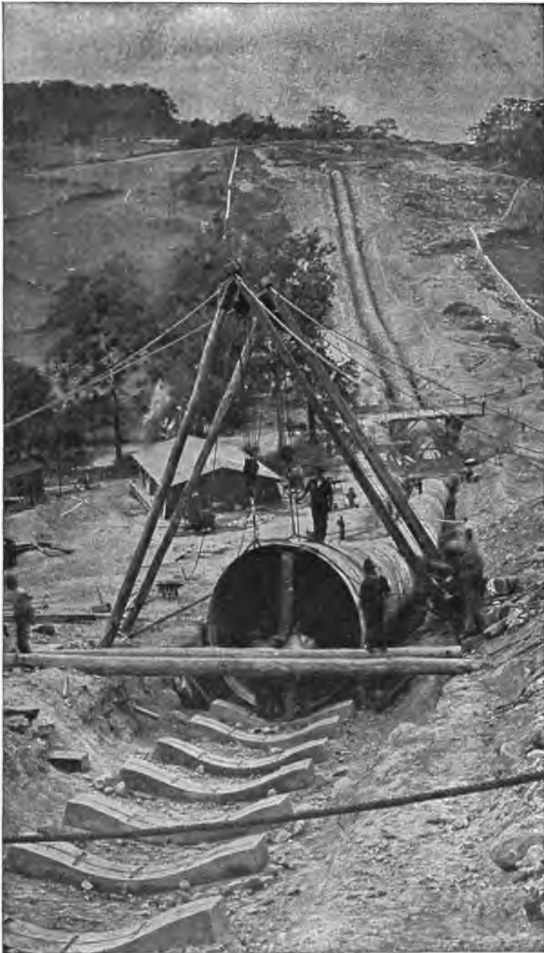
PLATE 159.—Contract 68. Hunters Brook Steel Pipe Siphon. Laying of steel pipe on concrete pedestal blocks. Later pipe was filled with water, covered with concrete and earth and lined with 2 ins. of mortar.
